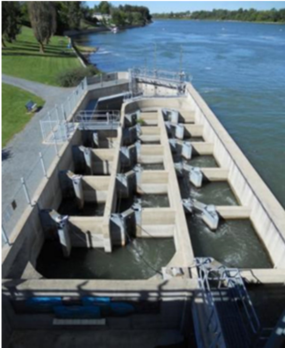
Fig. 3 The vertical slot fishway at the Vianney-Legendre fishway on the Richelieu River, Canada. Photo credit: Cooke Lab
